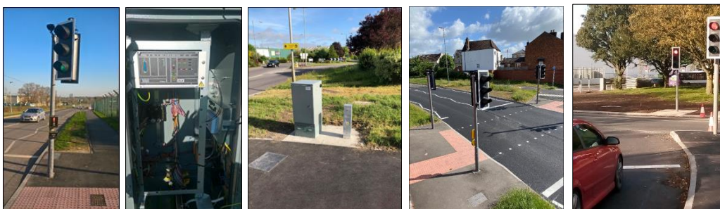
The traffic signals contractor Telent continued to maintain the equipment though out the year with the support of Atkins
