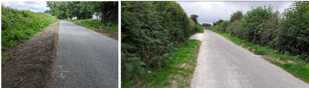
Verge and carriageway repairs were made to address damage by vehicles over running the verge on rural roads
