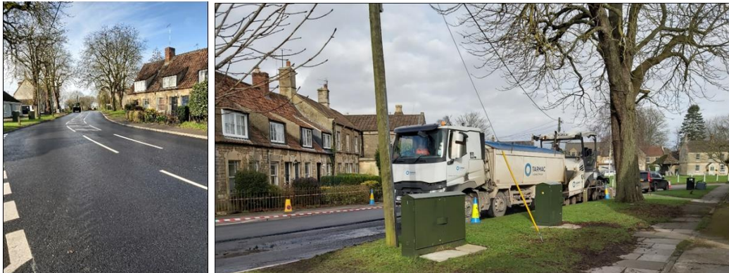
Tarmac resurfacing work continued through the lockdowns to ensure safe delivery of the road resurfacing programme
