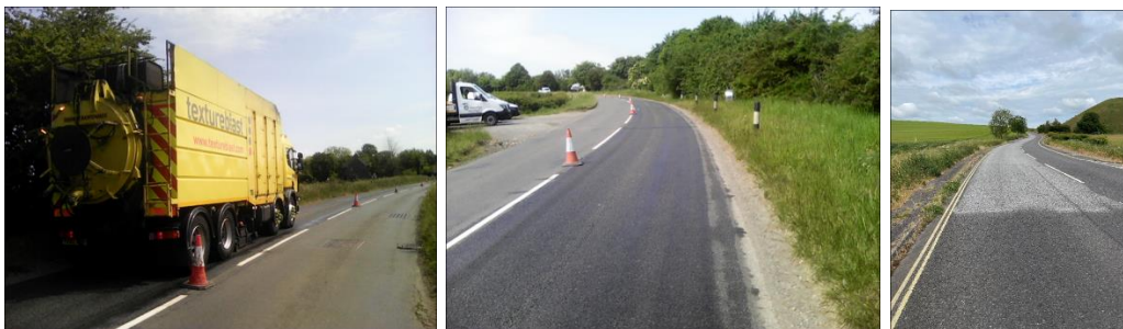
Road retexturing was carried out to restore skid resistance to carriageways at key locations, particularly at bends
